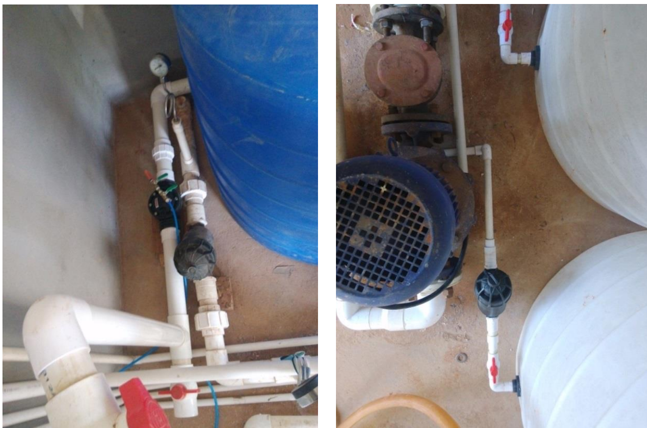
The input water line, irrigation pump and filters for input and fertilizers.
