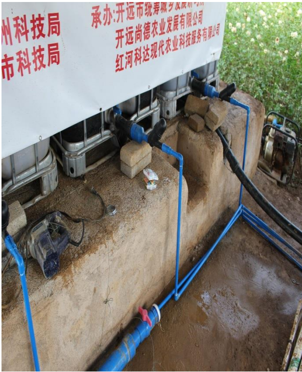
The fertilizer tank and the filters for each tank.
