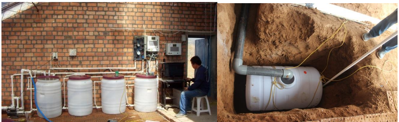
The full installed system
