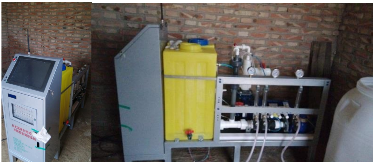
The full installed system.
