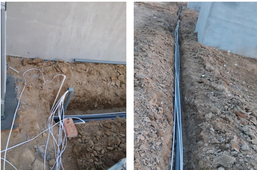
The water and wire lines.
