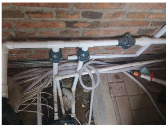
Two irrigation line
