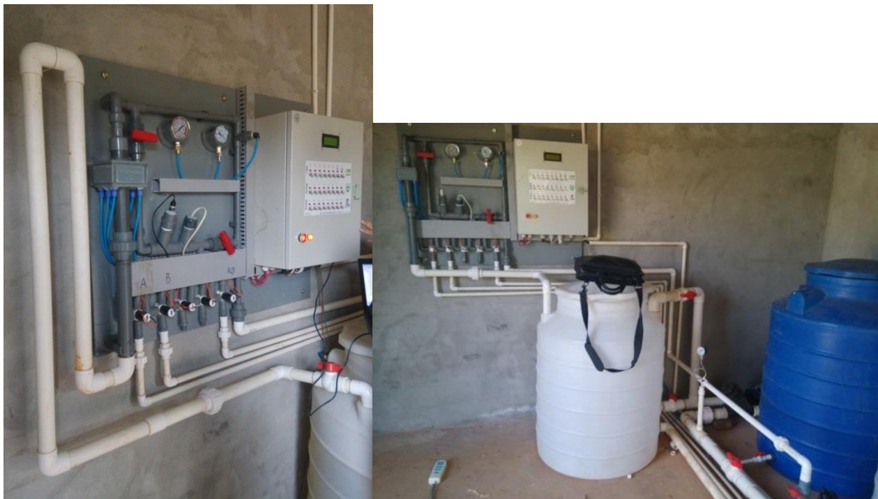
The full installed system.
