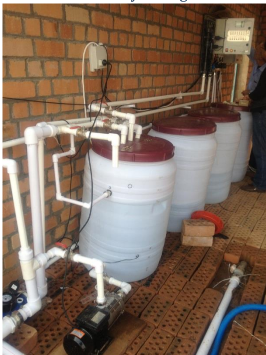
The fertilizer tank and irrigation pump.
