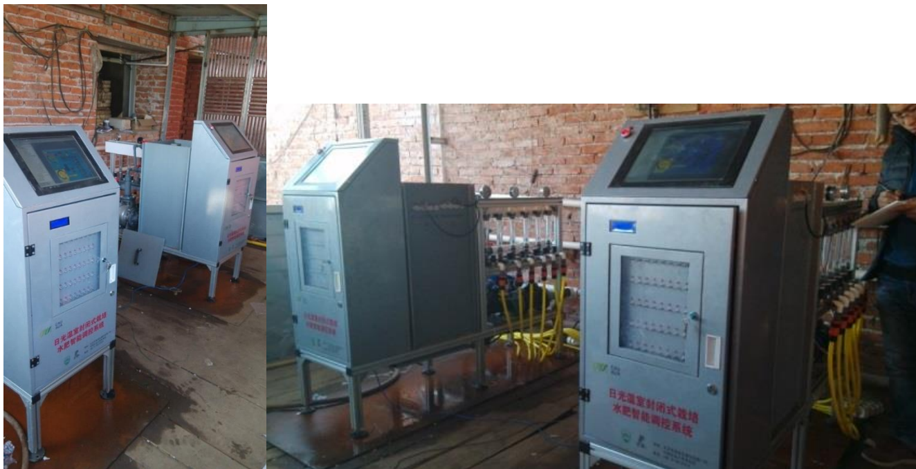
The full installed system.
