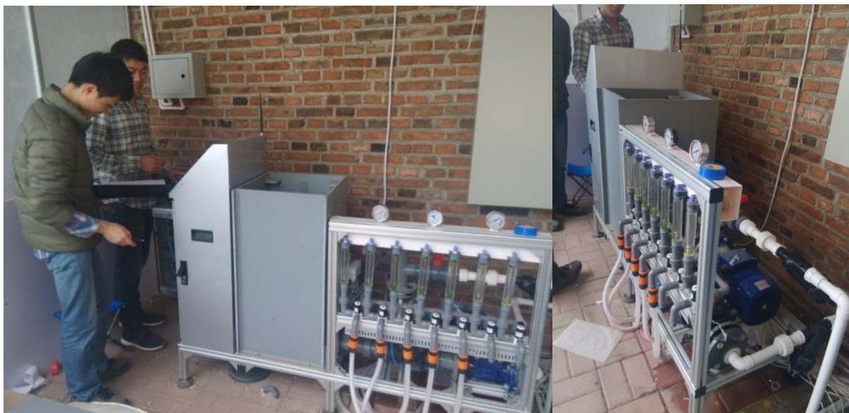
The full installed system.
